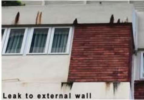
Leak to external wall
