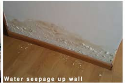
Water seepage up wall
